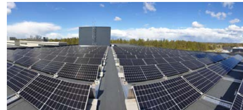
Photo: Solar panels at the Swedish Plant
