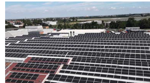
Photo: Solar panels at the Italian Plant
