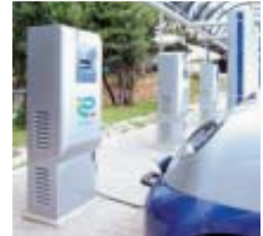
Battery Charging System for EV
