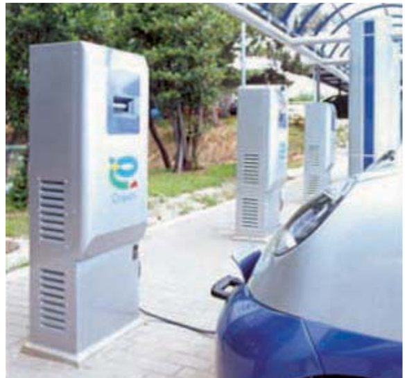
Battery Charging System for EV
