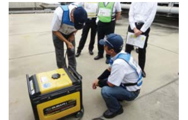
Confirming procedures to activate an emergency power generator
