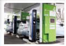
Smart Charging System Efficiently charges multiple plug-in hybrid vehicles and electric vehicles
