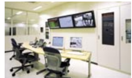
The machine room oversees the network connecting Toyota Industries' bases all over the world
