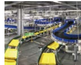
BHS (Heathrow Airport)
