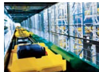
Baggage handling system in airports
