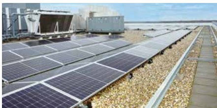
Rooftop solar panels installed by Vanderlande
