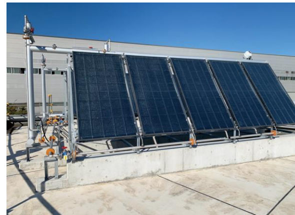
Solar heat collector
