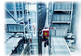
Bucket type Automatic warehouse
