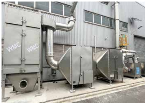
VOC collection and treatment equipment
