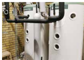
Heat storage tanks
